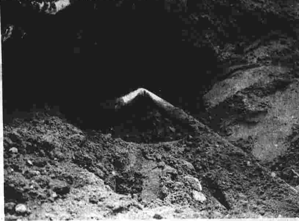
A gas line at East Center and Walker streets was broken Wednesday afternoon during installation of a new sewer line. The service line, which carries gas from the main line under the street to a customer, was broken by a shovel digging a path for installation of the sewer. The town fire department notified Connecticut Natural Gas Corp. of the break about 3 p.m., and representatives quickly repaired it, according to a fire department spokesman. Louie Stoppa, a public affairs administrator for the gas company, described the break as "a very minor problem." (Herald photo by Pinto)
